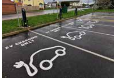
EV Chargers, Lynnsport
